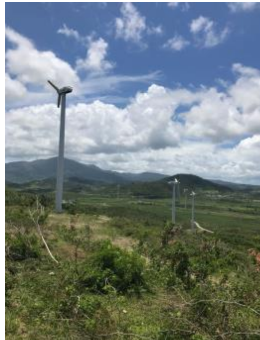
Figure 1: Damaged turbines at Punta Lima Wind Farm After the Passing of Hurricane María
