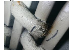
Figure 1.3 Corona discharge tracing in overhang end winding
