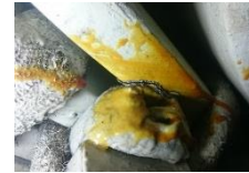
Figure 1.2 Greasing compound in end winding ties
