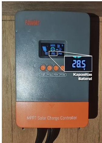
Figure 9. Results of charging the battery using the solar tracker
